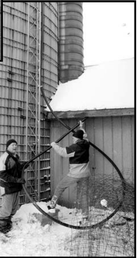
LEFT: TOM RICHMOND AND DAYLE GOWAN PREPARE THE END OF THE 1 5/8-INCH COAX CABLE TO FIT THE TRANSMITTER.
